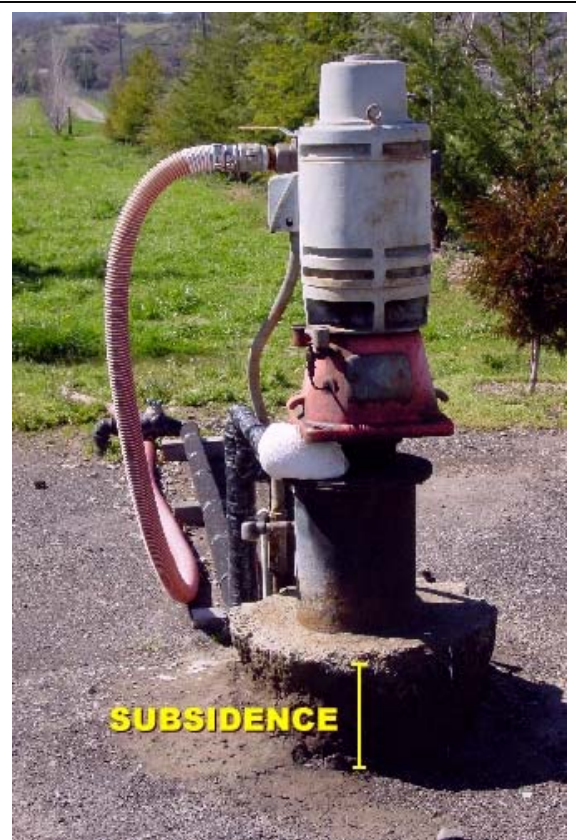
A groundwater well along Scotts Valley Road, showing subsidence around the well collar.
